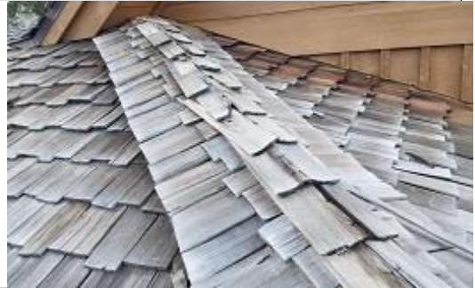
Ridge tiles broken and missing
