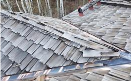
Many broken shake tiles
