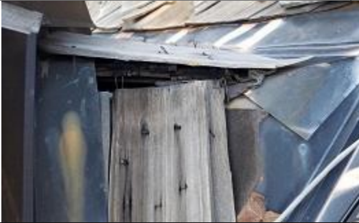
Holes in roof, this one in a valley apex
