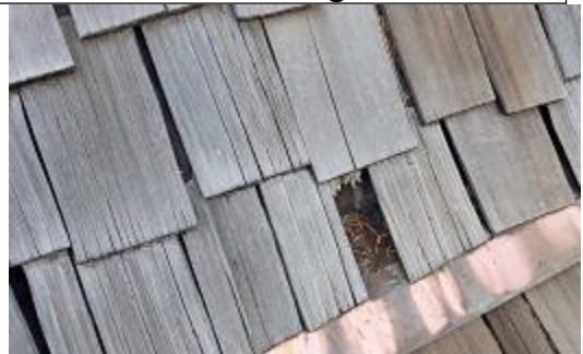
Holes in roof
