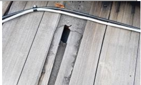
Holes in roof
