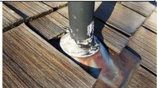
Cracked pipe jack
