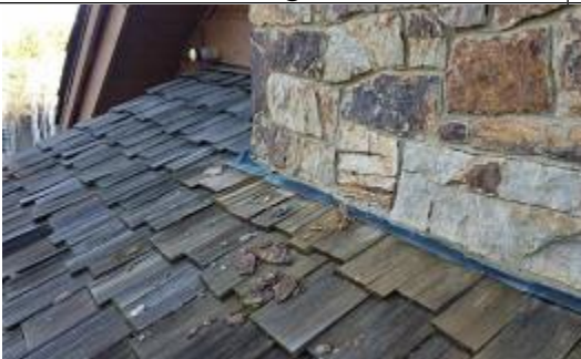
Crumbly chimney stone
