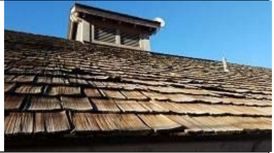
Overview of south slope (minor cupping)
