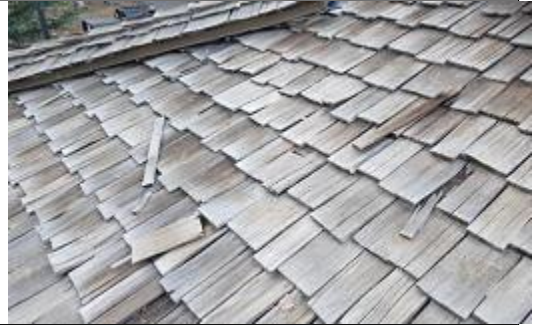
Many broken shake tiles
