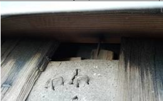
Holes in roof (under headwall)
